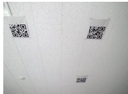
Fig. 2 QR codes stuck on the ceiling
